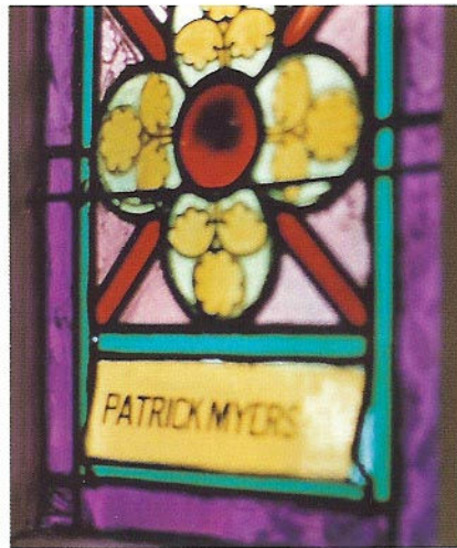
Buckling is so severe in this window, that the dedication plate is falling out.
